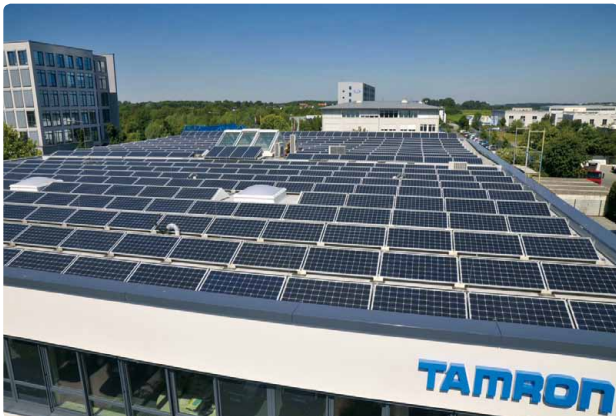
Rooftop PV panels at Tamron Europe GmbH
